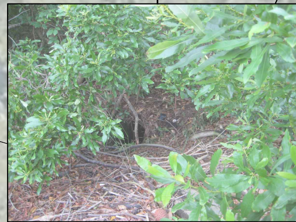
OUTFALL 24" CMP HALF FULL OF DEBRIS
