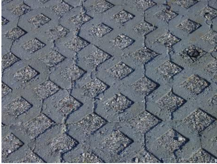
Pervious paving infiltrates stormwater back into the soil thereby recharging groundwater.
