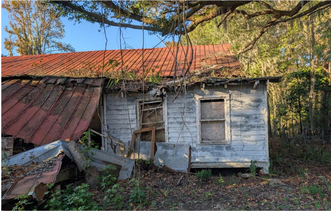
Right Rear Showing Deterioration
