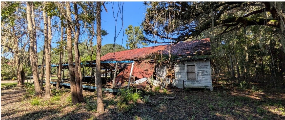
Right (Looking Northwest) Overall Showing Deterioration
