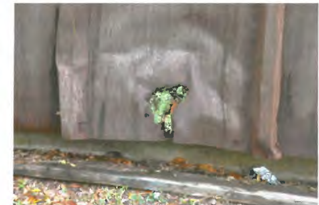
Above: Rusting, warped exterior.
