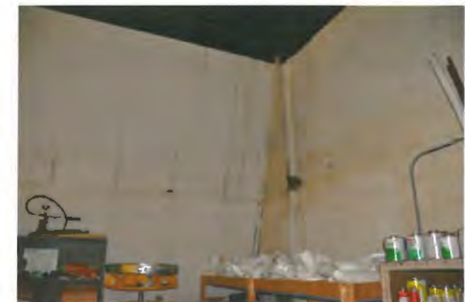
Above: Deteriorating, aged interior.
