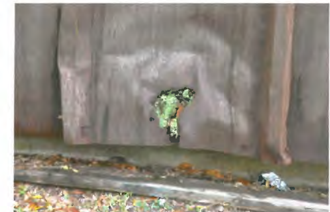
Above: Rusting, warped exterior.
