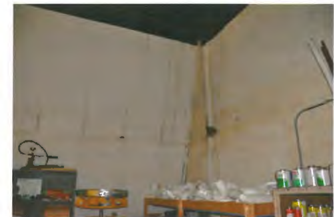
Above: Deteriorating, aged interior.
