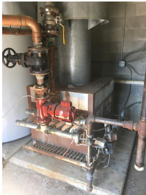
Existing Domestic Boiler
