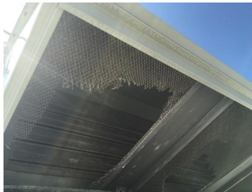
Corroded Birdscreen on RTU
