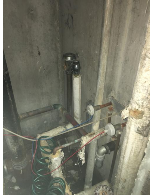
Existing Piping in Chase
