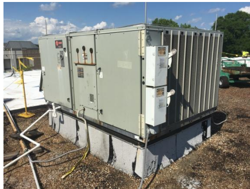
Existing Rooftop Unit
