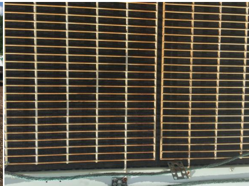
Corrosion on Condenser
