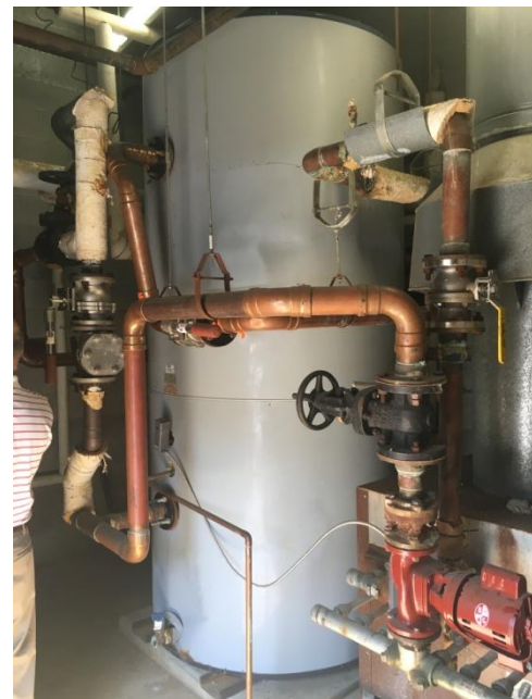
Existing Storage Tank
