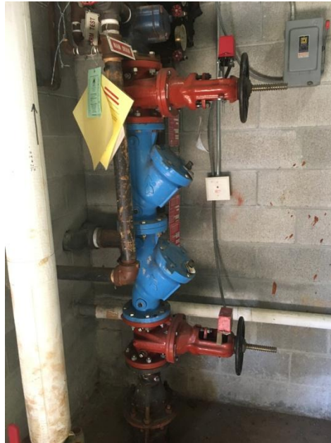
Existing Fire Service and Backflow Preventer
