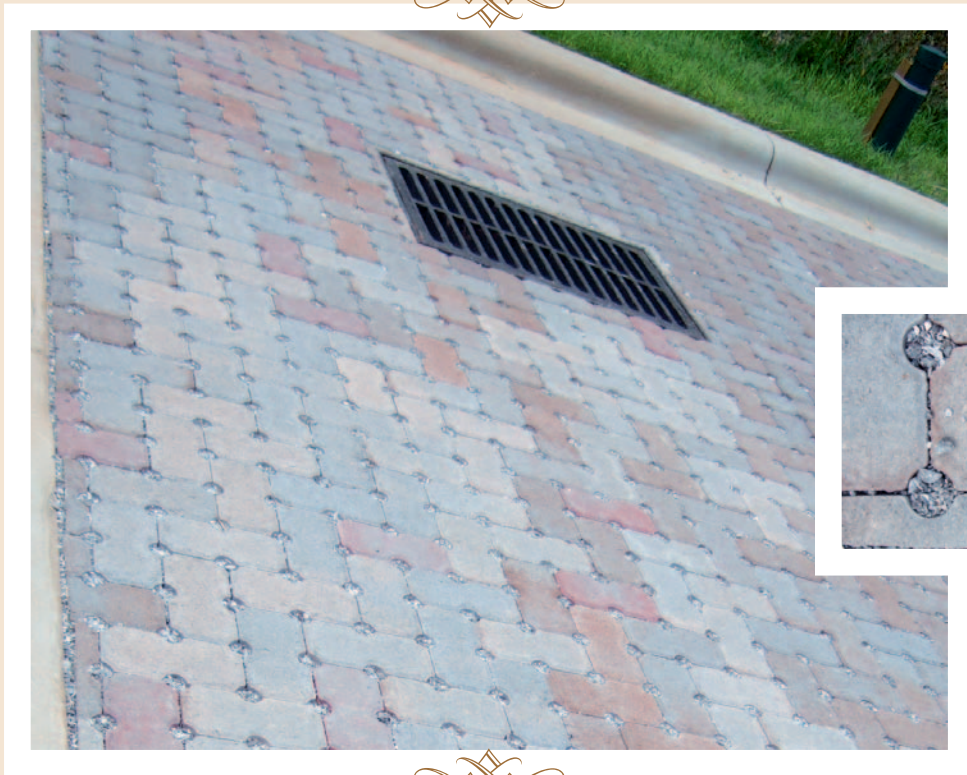
An example of a block paver parking lot. The pavers allow for stormwater to flow into a porous gravel substrate to be collected and routed to a natural treatment area such as a rain garden or created wetland (described later).
