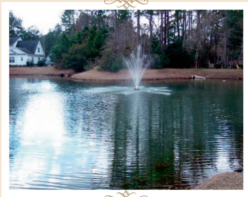
An example of a fountain aeration system installed in a stormwater pond.
