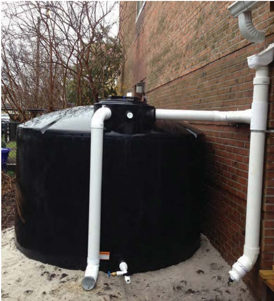
Figure 4.23. Example cistern application (photo: Marty Morganello).
