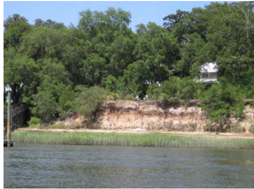
Image 9. Bank erosion along the May River.
