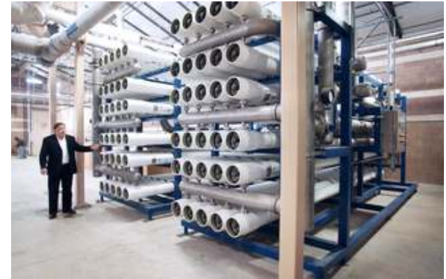
RO filter skids
