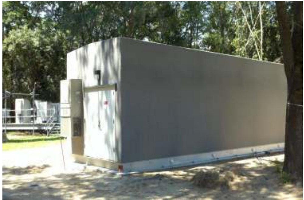
PSD Water Booster Station at Wildhorse Tower
