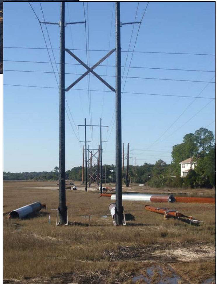
Final Four Power Poles to be replace along the Proposed 5A Project Area
