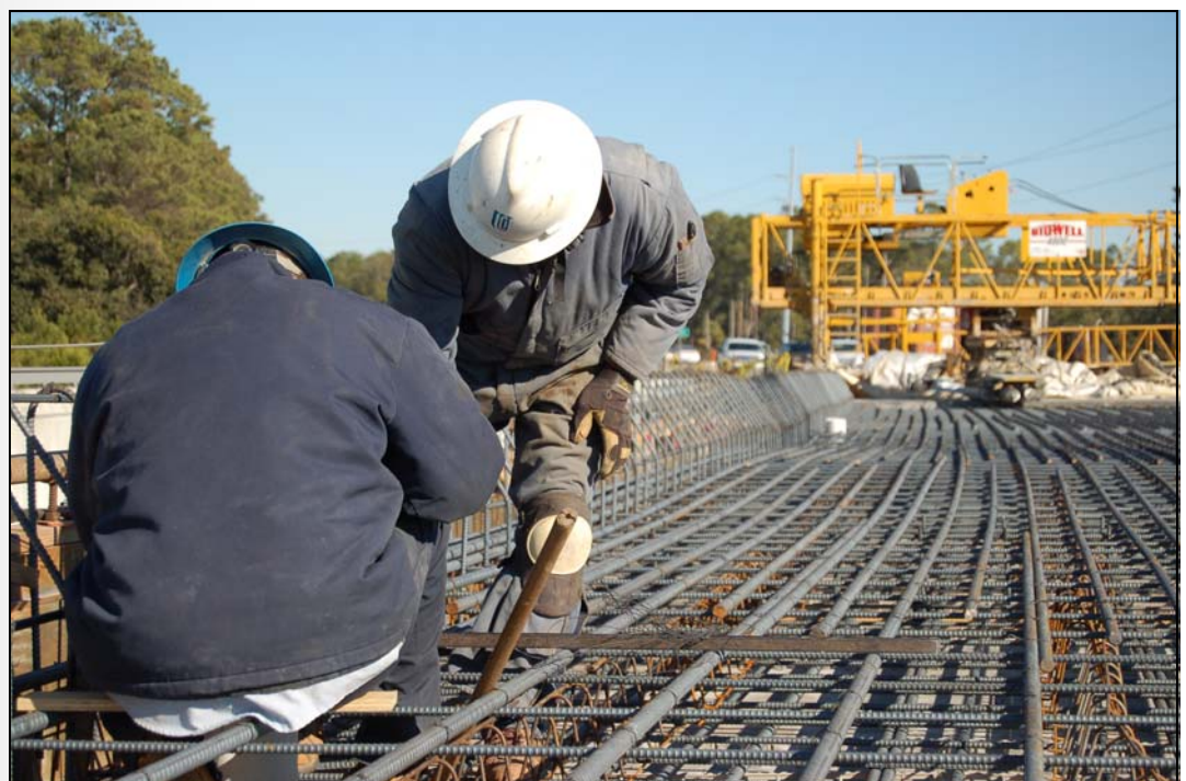
United Contractors' Employees Working on the Bridge Deck Reinforcing Steel for the New SC 802 Bridge
