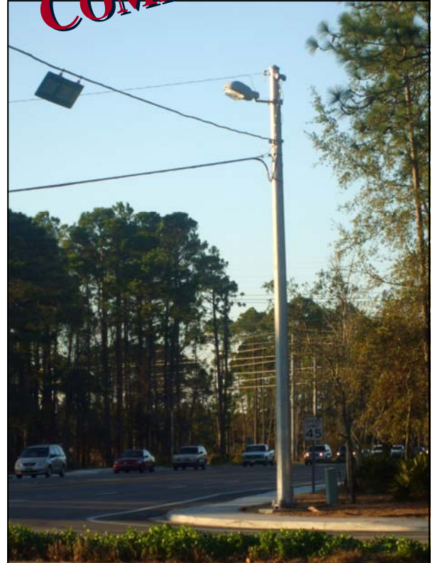
Newly Installed Street Light Fixture
