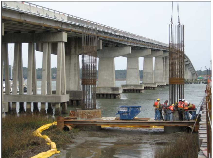
Drilled Shaft Crew Placing Rebar Cages on the West End of the New SC 802 Bridge
